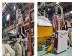
Local Preheating system
