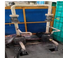
Reservoir for pump suction line
